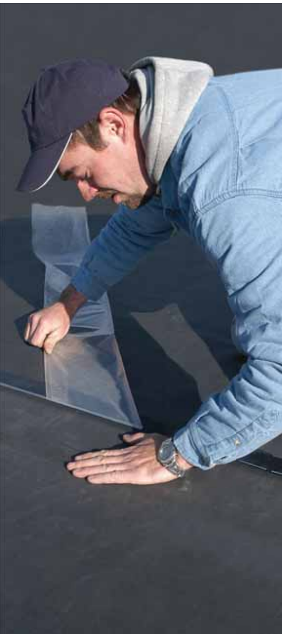
Seams completed with WeatherBond Pre-Applied Seam Tape go together smoothly resulting in fewer wrinkles.
