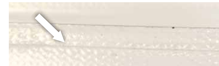
INCORRECT. HEEL DRAG CAN CAUSE DAMAGE TO MEMBRANE.
